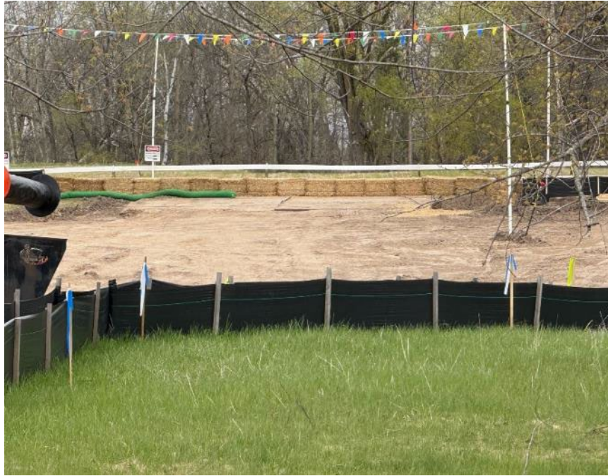
Facing east near MP 2.3, certified weed-free straw bales installed at the access road to enclose the temporary workspace and exclude Blanding's turtles
