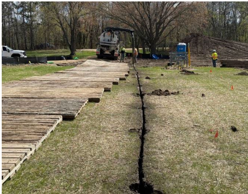
Facing south near MP 2.39, InterCon conducting hydrovac to locate the utilities prior to construction
